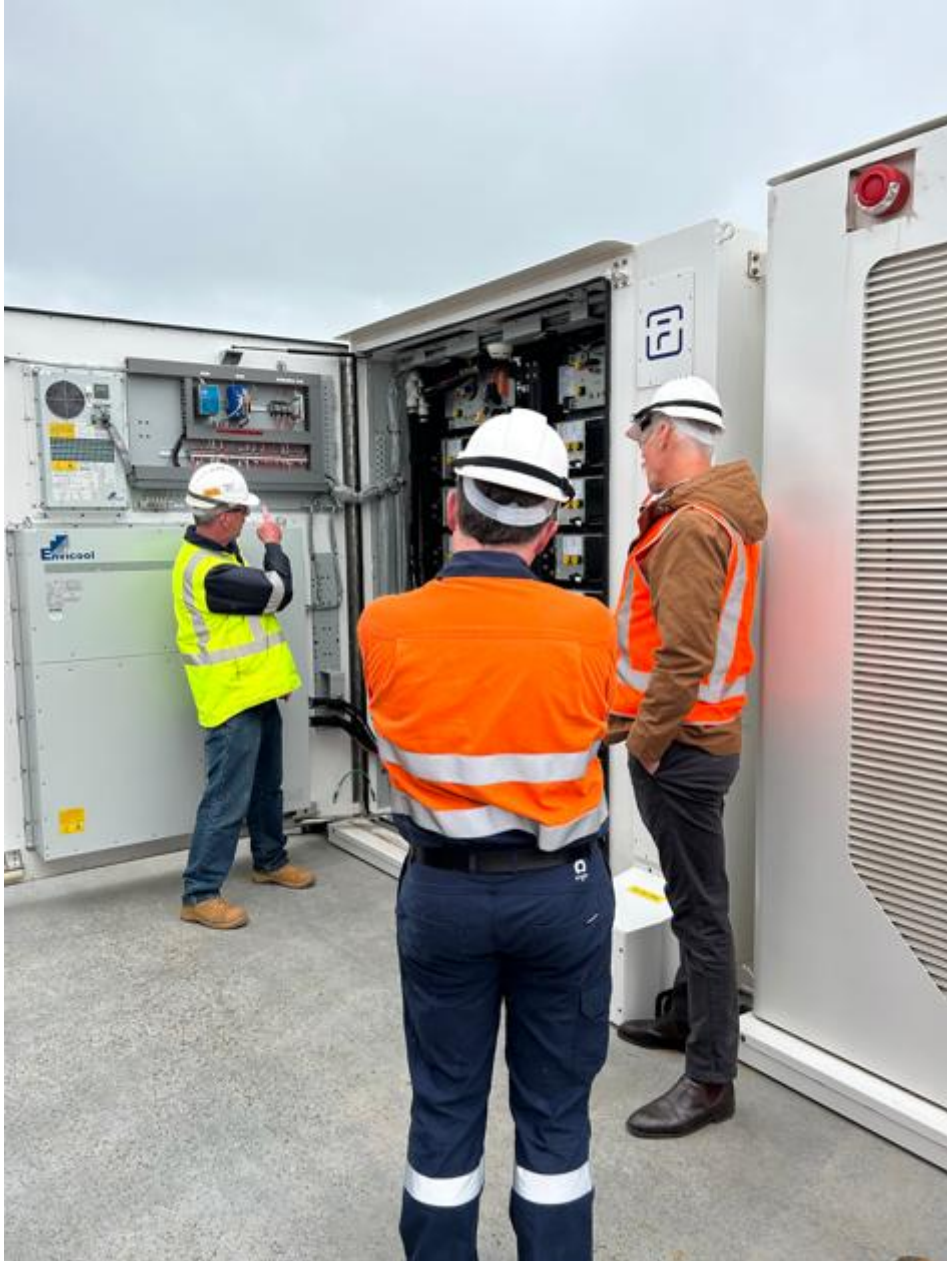
Visiting a grid-scale battery facility
